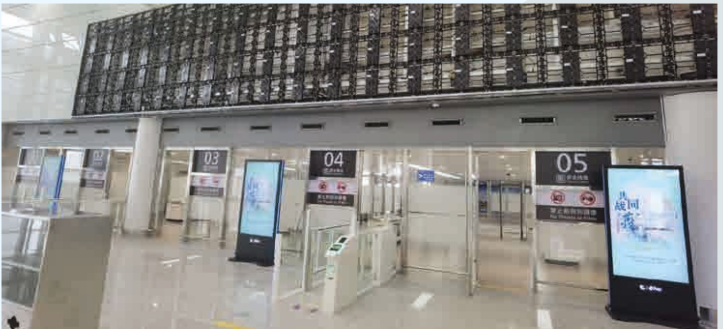
In the photos some details of the new installation of ABC GATE in Nanjing.
